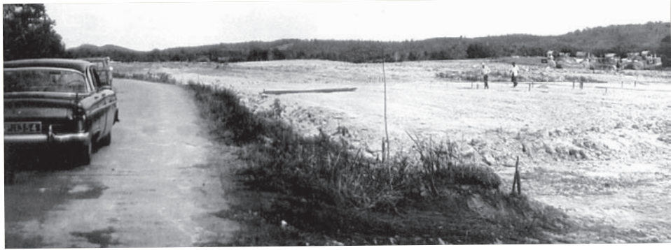
Just after the dozers cleared the farmhouses and vegetable plots to make way for the first buildings of SAFTI. View from Pasir Laba Road from the spot where the main gate would come up.
